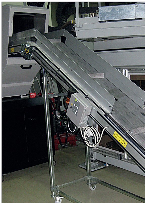
Installation example: Machinery protection. Plate type metal detector ELCON installed on the conveyor belt leading to the granulator. (old version)
